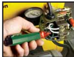
Control panel troubleshooting
